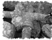
THESE PIPES ARE IN THE MIDDLE OF CHEMICAL CHANGES AS THEY RUST.
